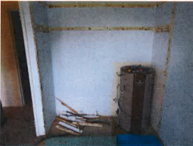
Figure 9: Photo of the electric hot water service to be replaced with gas
